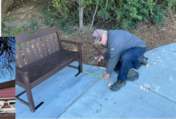
Millbrae Dept of Public Works employee - Noel Gantley, installing bench #3 @ Josephine Waugh Soroptimist Park.
